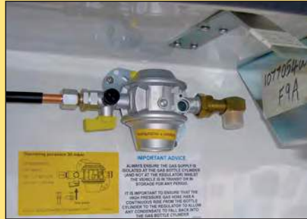
Truma Regulator already supplied with a 90 degree elbow fitted on its side close to a reinforcing strut
