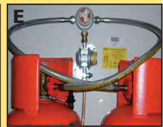
Picture shows a Truma regulator upgraded to an Auto changeover with a 01-1755 and using two propane 0.75 meter Stainless hoses. Note how the hoses cross preventing unnecessary kinking and twisting.
