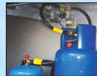
A twin system with a 0.45m and 0.75m rubber hose using a Gaslow Manual Changeover Adapter (01-1626) connecting a Camping Gas and a 7kg Butane cylinder.
