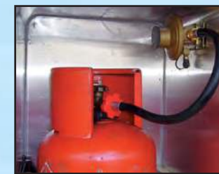
A single 0.45m EasyFit rubber hose system fitted to a Nova Comet 30mbar system.
