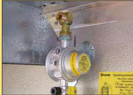
Truma Regulator already supplied with a 90 degree elbow fitted close to a reinforcing strut on the left
